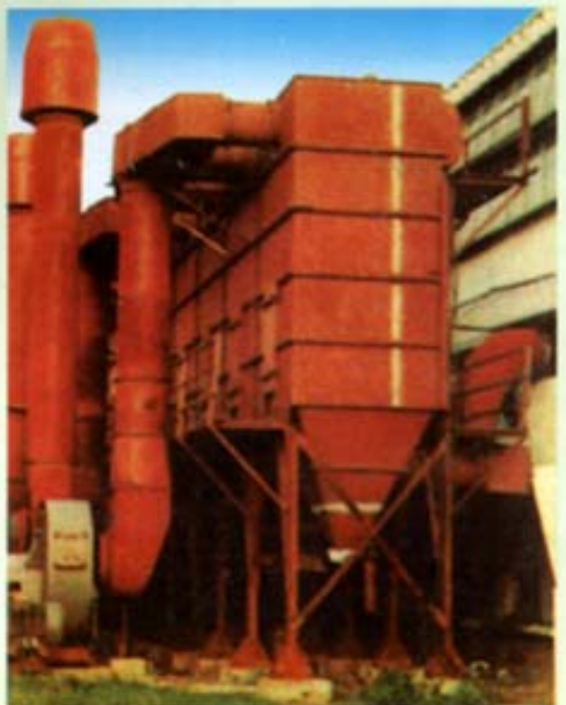
▲ Pulse Air Jet Bag Filter Installation.
